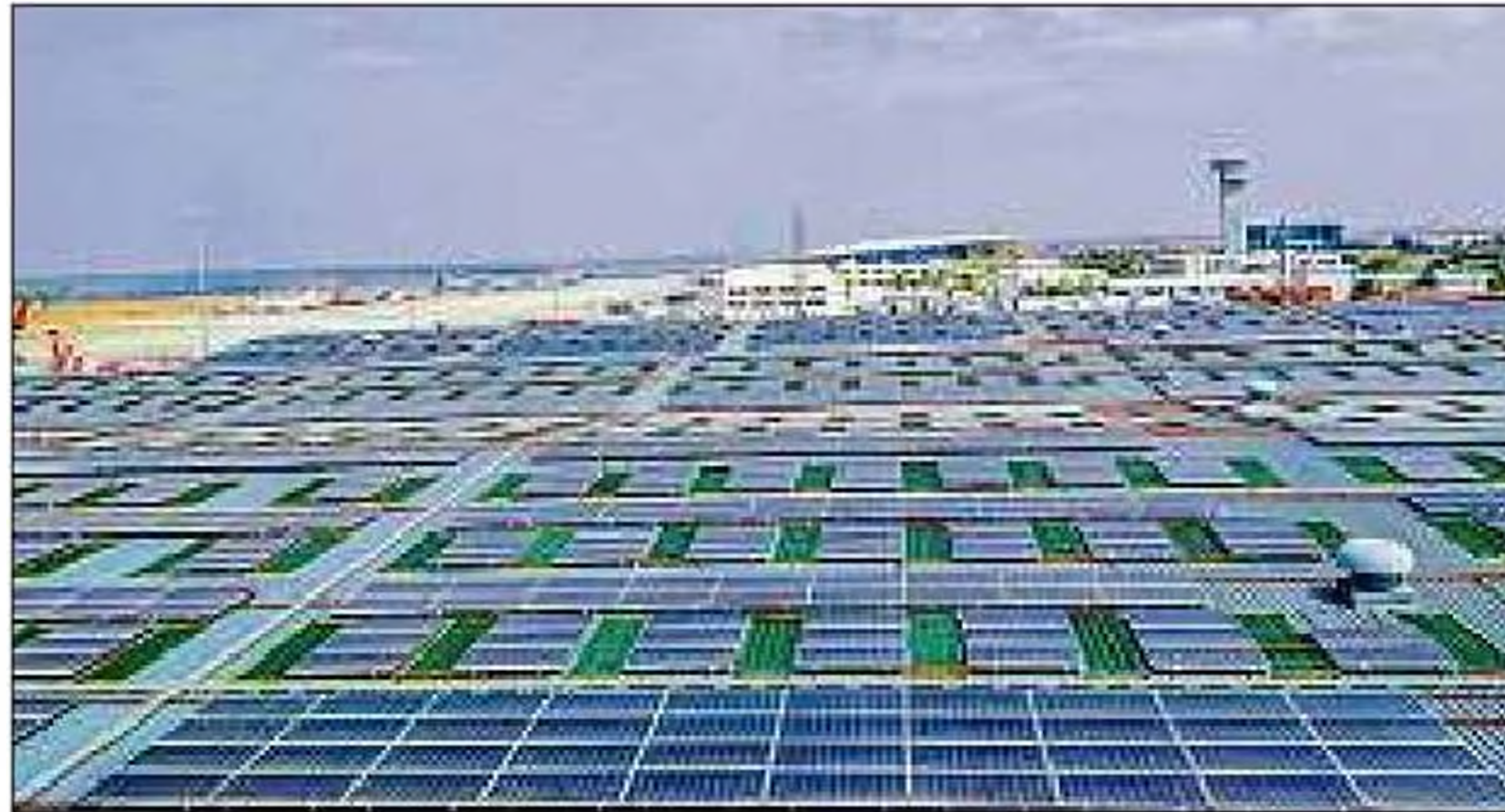
The solar panels installed on the rooftop of the Kempegowda International Airport.
